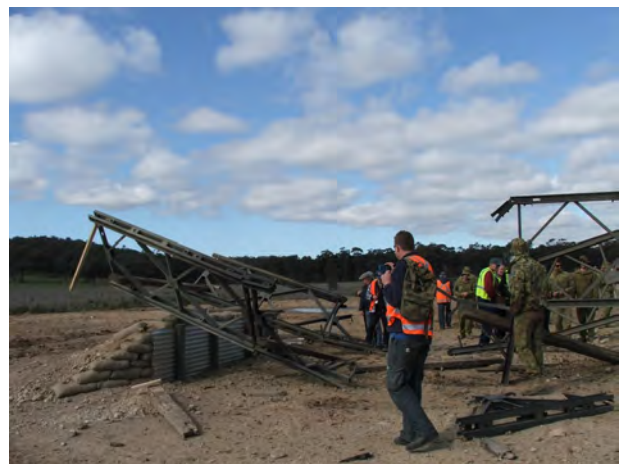
A Thoroughly Demolished Bridge Span
